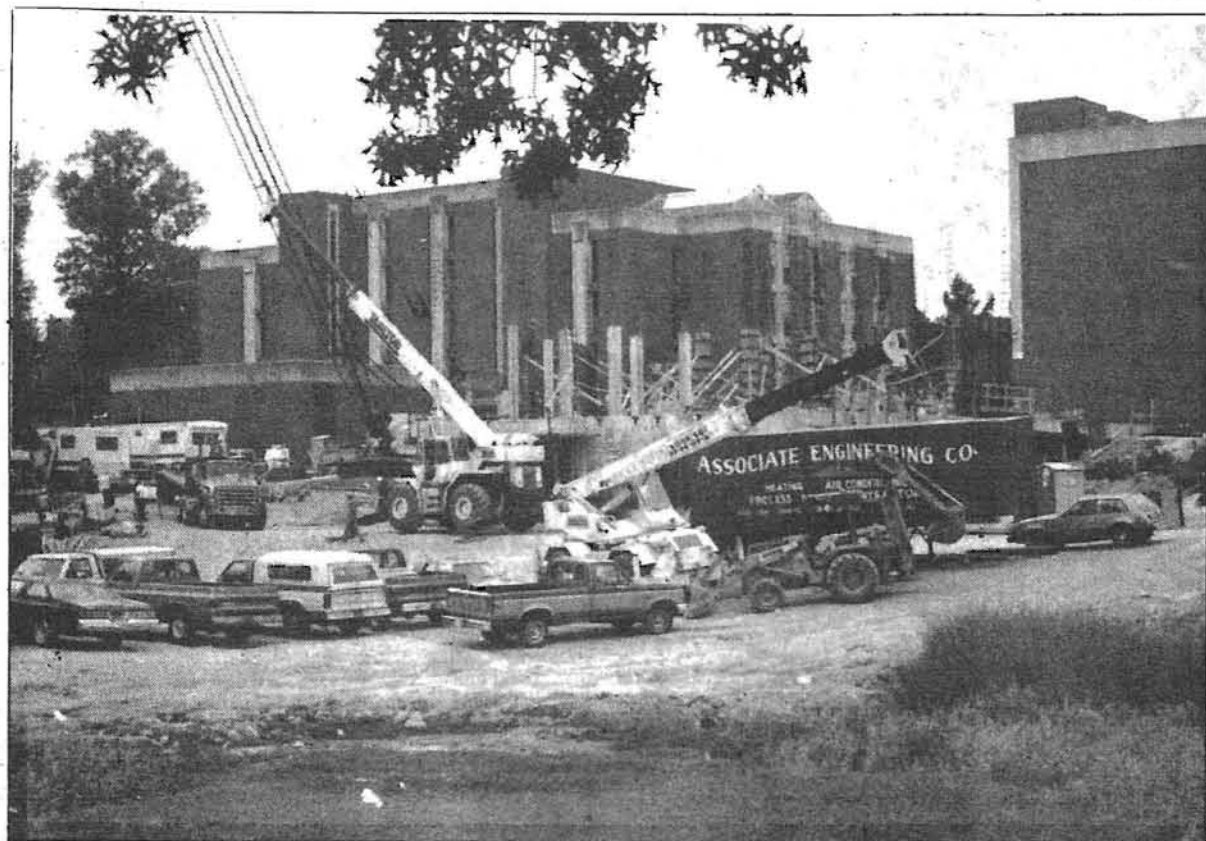
Construction on the new $19 million science complex continued throughout the year. More construction is scheduled for May when ground will be broke for the $6 million two-story addition to the library.
